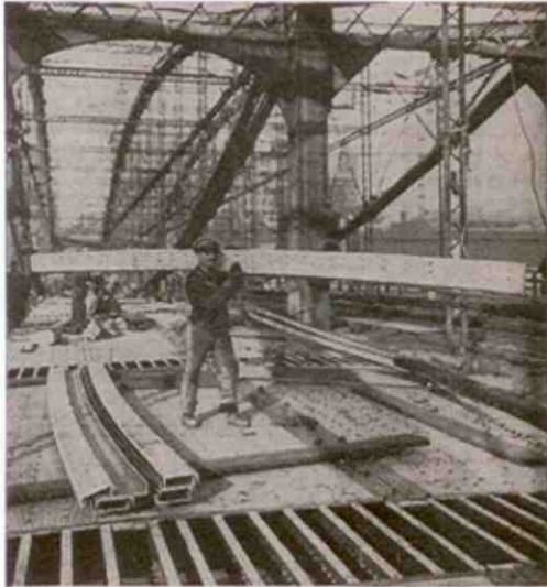
Huge aluminum girder is swung about with ease. Even today light metals replace steel in some structures.
