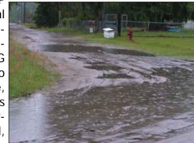
Seen above is one of the streets slated for improvement with CDBG funds in the City of Homeland. Upon completion of the project, residents will no longer be forced to navigate these dangerous road conditions.
